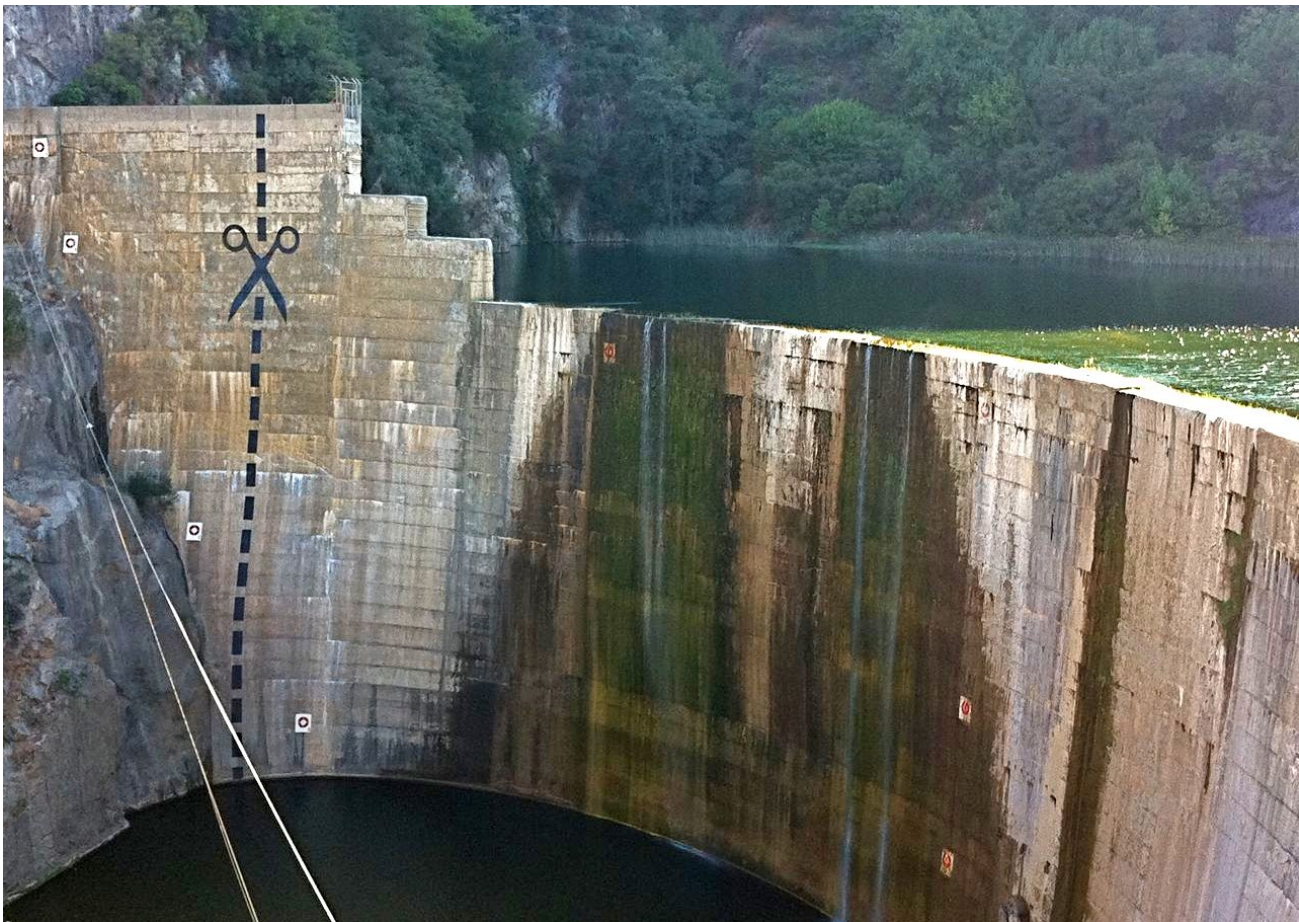
Matilija Dam Notches. The top of the dam was notched in 1965 and again in 1978 to address safety concerns, including strain on the dam from water stored behind the dam and deteriorating concrete. The original dam height was 198 feet and is now 168 feet (USACE 2004). In 2011, someone painted a huge pair of scissors and a long dotted line on the face of the dam.
