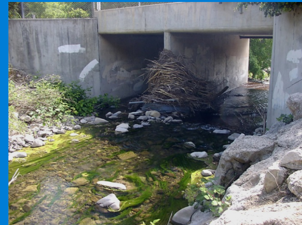
Boardman Road – San Antonio Creek
